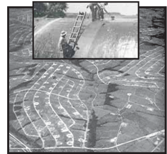
Igloos are solid concrete affairs covered with earth. When the igloos were built, each piece of metal used is grounded. They are safely spaced in case of explosion. Waterproofing igloos prevents possible moisture damage to stored ammunition.
